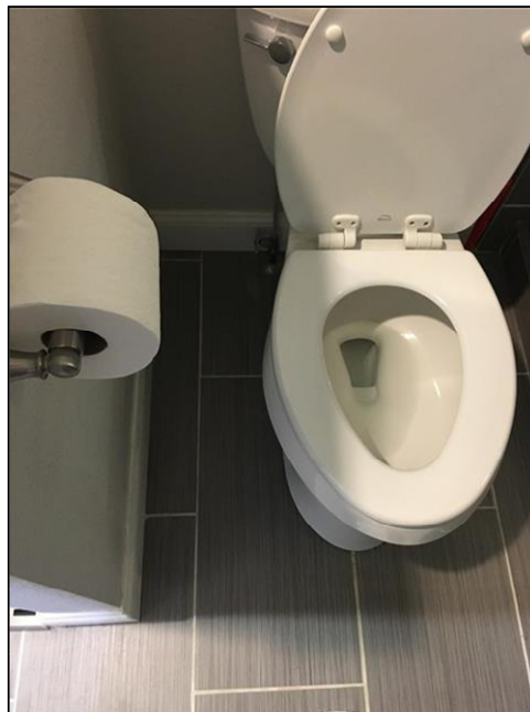
6.8 Item 2(Picture) loose master bath toilet
