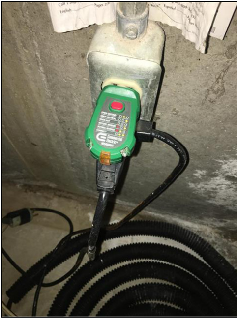
9.4 Item 1(Picture) non-working sump outlet
