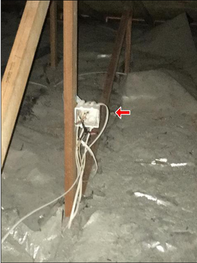
1.8 Item 1(Picture) open junction box
