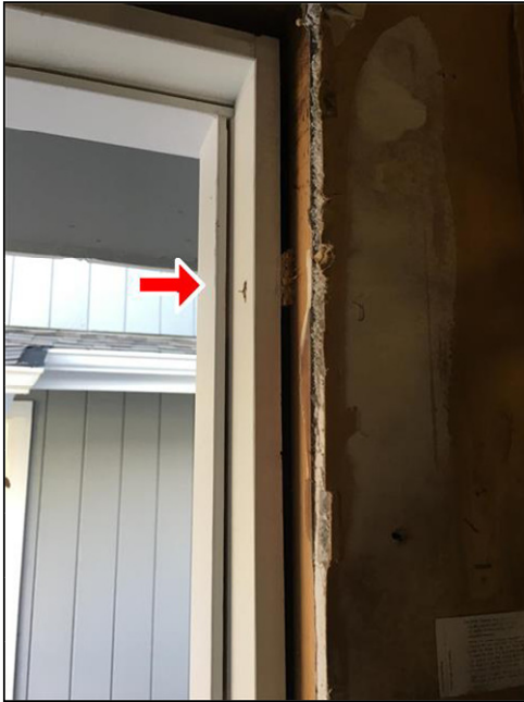
2.1 Item 1(Picture) missing weather stripping in garage service door
