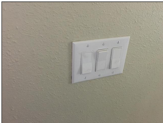
5.6 Item 1(Picture) loft/hallway switches
