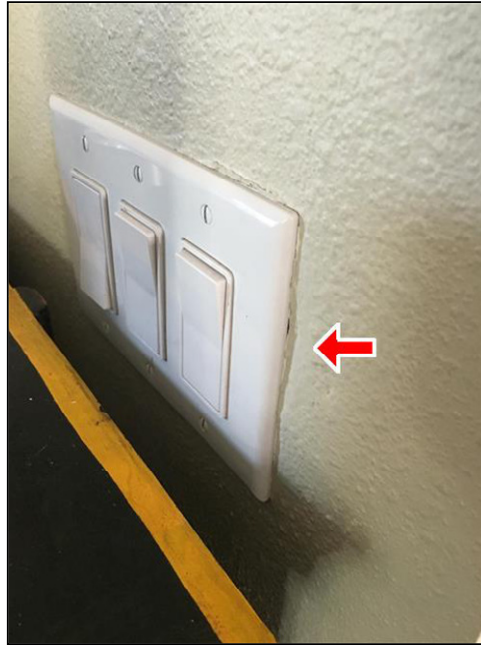
4.8 Item 2(Picture) kitchen switches
