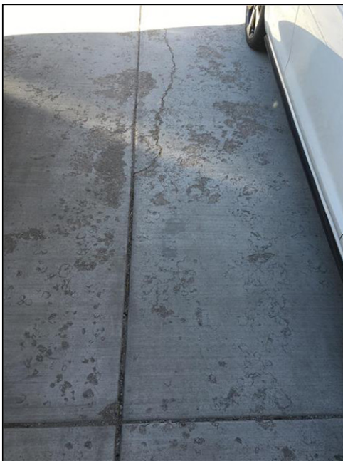
2.4 Item 7(Picture) flaking concrete
