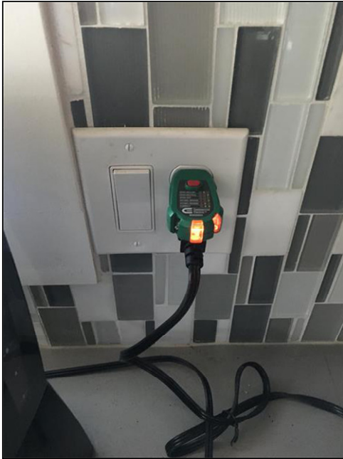
4.8 Item 1(Picture) non-protected gfci outlets
