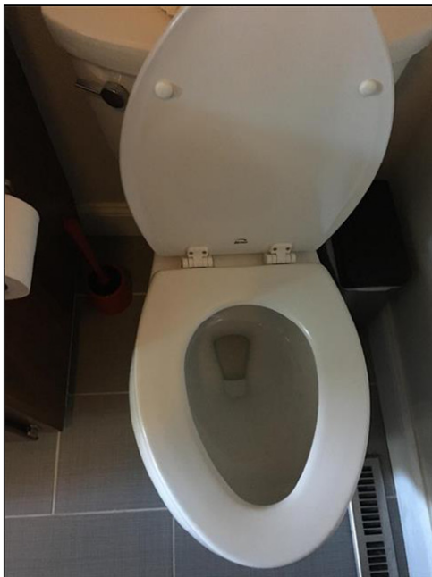
6.8 Item 1(Picture) loose toilet-main bath
