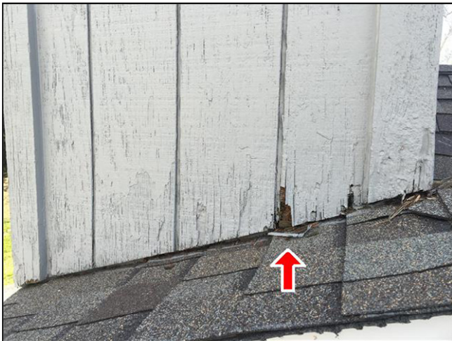
2.4 Item 3(Picture) deteriorating siding on the chimney
