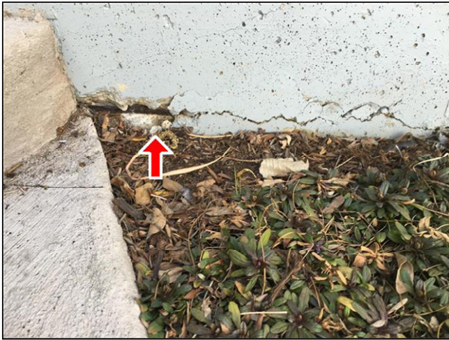
2.4 Item 5(Picture) Deteriorating concrete, exposed rebar
