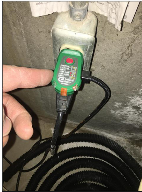
9.4 Item 2(Picture) working sump outlet when pressure is applied
